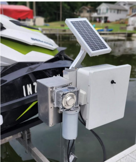
Example of finished installation on vertical lift
